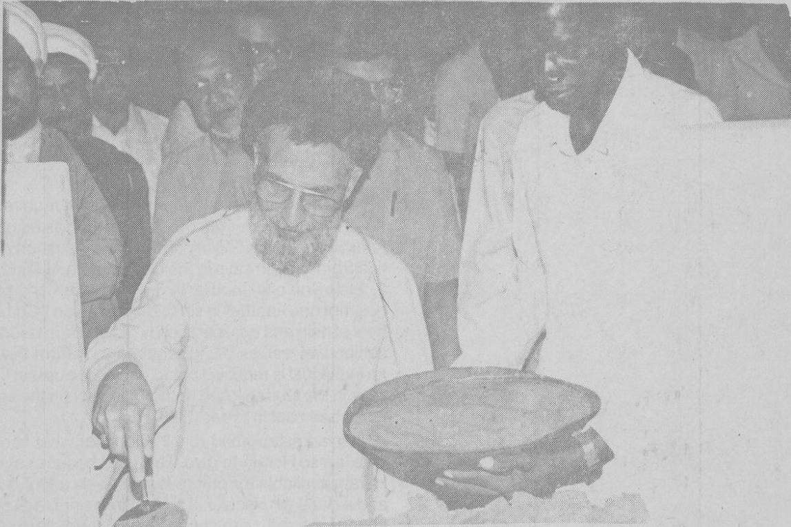
Hujjatul-Islam Syed Lavasani laying the foundation of the proposed extension of the Al-Muntazir Islamic Seminary. The chairman of the Federation, Habib Mulji and President of Dar es Salaam Jamaat, Aliraza Rajani (partly hidden) are on the background.
